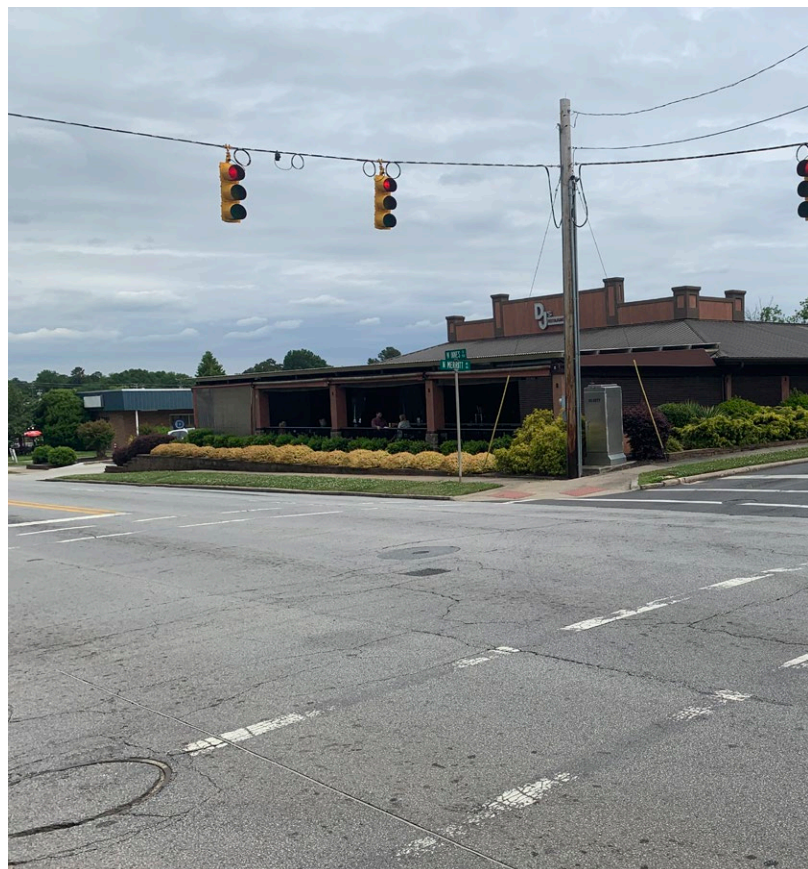
Intersection in Salisbury, NC with faded crosswalk markings
